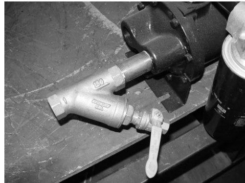
Figure 4 Wye-strainer installed, with cleanout valve.
