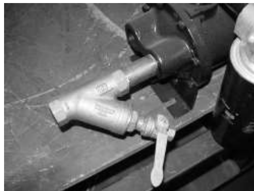
Figure 5 Wye-strainer installed, with cleanout valve.
