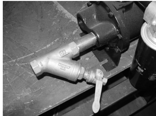
Figure 12 Wye-strainer installed, with cleanout valve.
