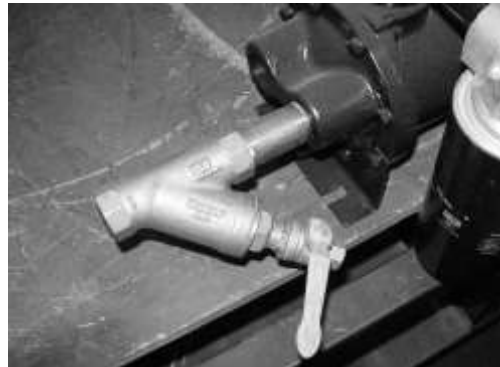
Wye-strainer installed, with cleanout valve.
